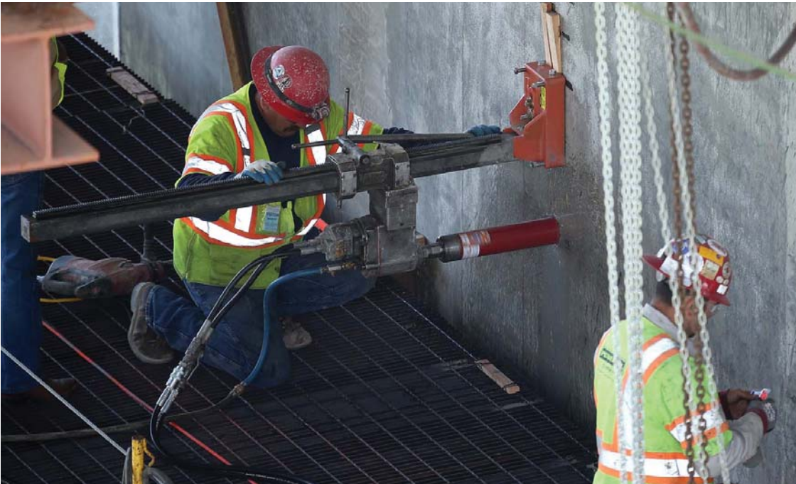
A worker drills into concrete on the underside of the newly constructed San Francisco-Oakland Bay Bridge on May 23, 2013 in Oakland, California. Bridge workers began installing large steel saddles over two seismic safety devices on the new East Span of the San Francisco-Oakland Bay Bridge to fix a problem with broken bolts on two shear keys. Justin Sullivan/Getty Images
